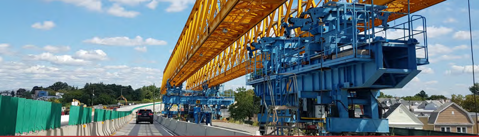
A Balancing Act - Bringing the Bayonne Bridge into the Modern Age, McElhanney, New Jersey, USA
