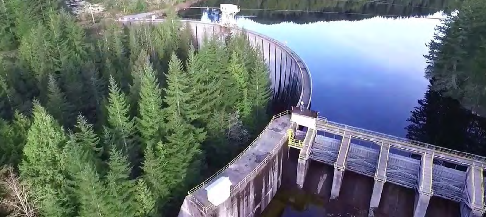
Lois Lake Dam Structural Evaluation, Klohn Crippen Berger Ltd., Powell River, BC
