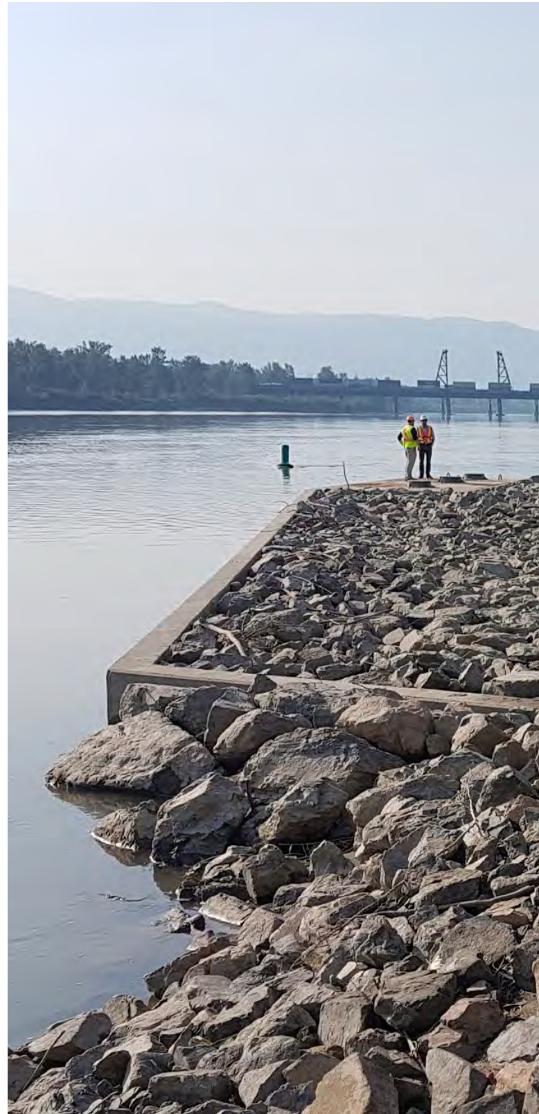
North Thompson Emergency Water Intake, WSP, Kamloops, BC
