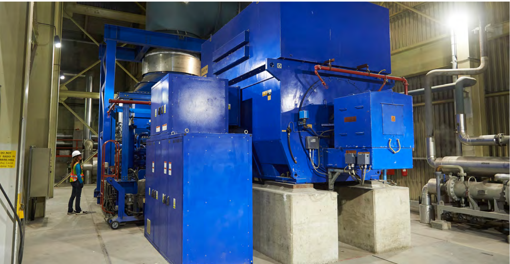
Protecting Public and Environmental Health - Metro Vancouver Waste-to-Energy Facility, HDR Corporation, Burnaby, BC
