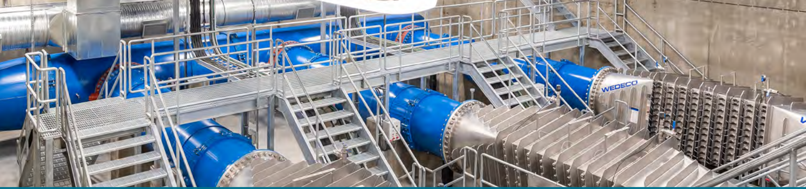
Greater Vernon's Water System - An Innovation in UV Disinfection, WSP Canada, Lavington, BC
